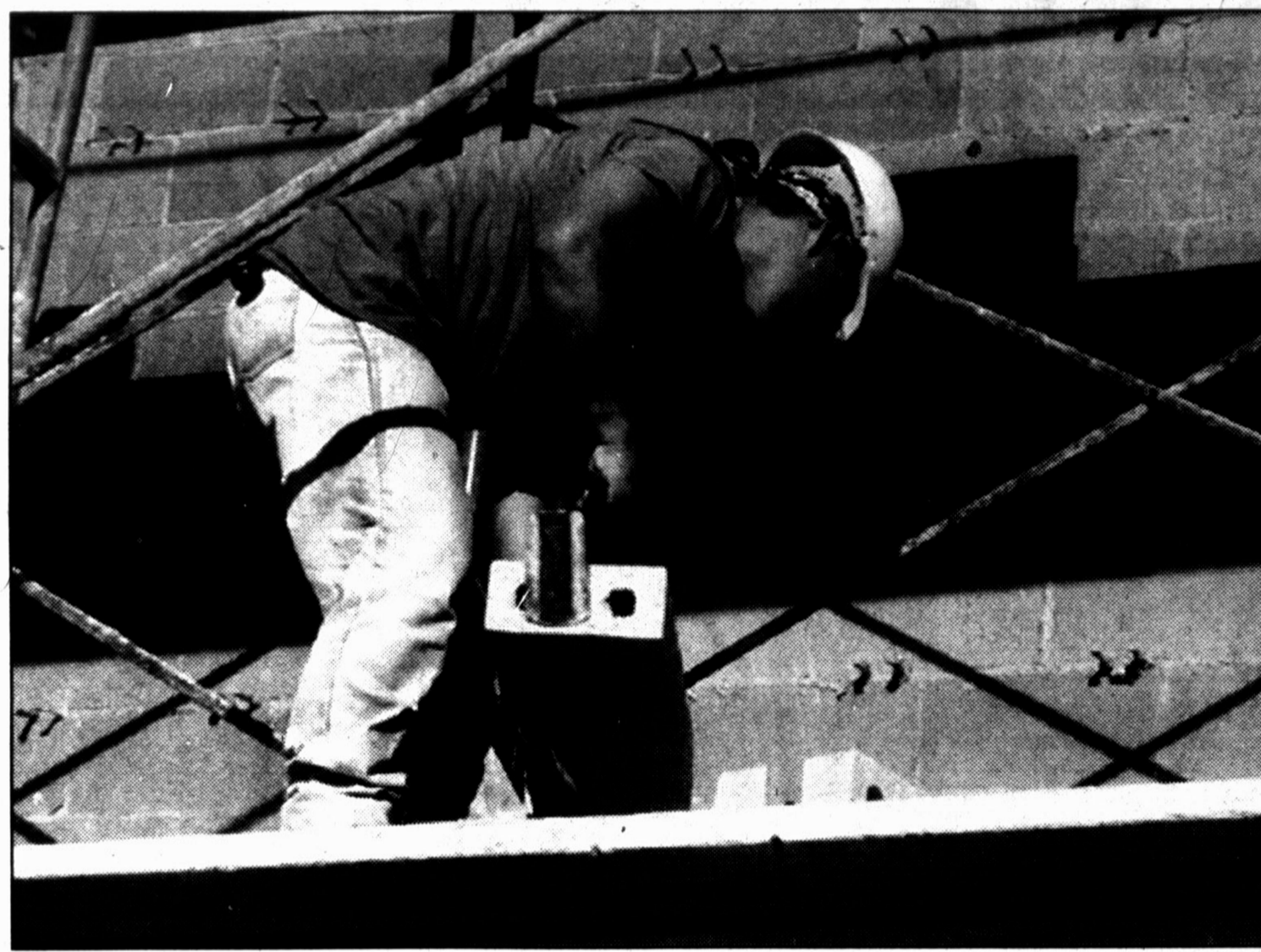
Moving bricks — The Fine Arts Center expansion at Hereford High School is nearing completion. Ricky Trevino, a brick layer, readies piles of bricks early Thursday prior to beginning the day's work. The bricks on the new building closely match the bricks of the existing buildings and should be nearly an exact match with the passage of time. The fine arts center should be ready for use shortly after the new school year begins.
