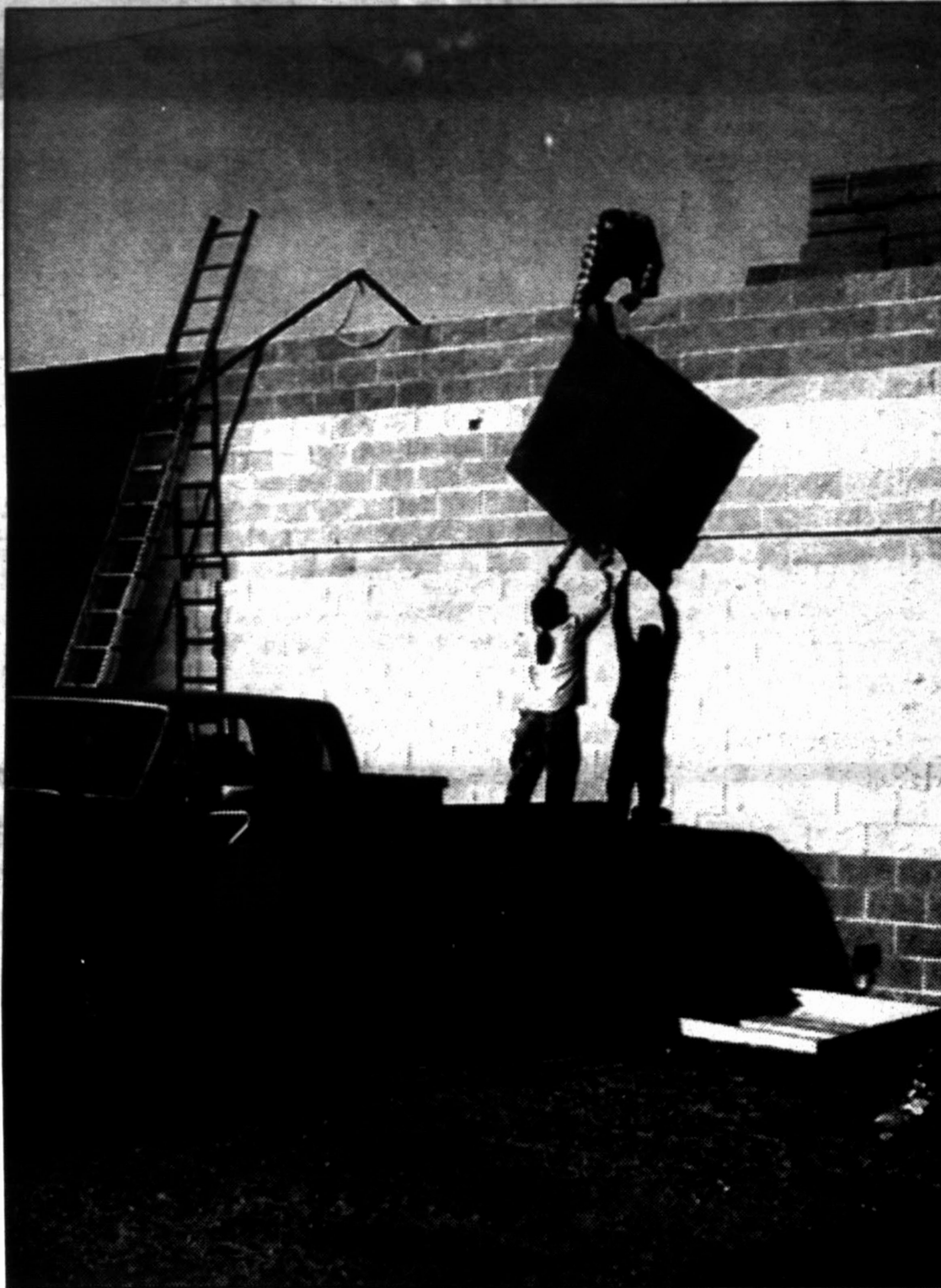
Going up — Wherever drivers look, they can see the signs of ongoing construction like these workers handing up roofing supplies at the new convenience store near the intersection of U.S. Highways 385 and 60.
