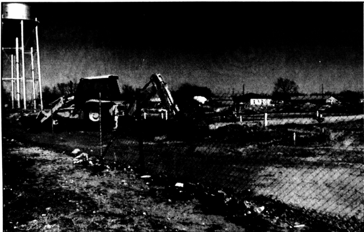
Constructing education — Additions to the Hereford Independent School District, and the High School campus in particular, continue to move forward. Workers move dirt, readying the area for more foundation work on the planned Tech/Prep facility north of the high school.
