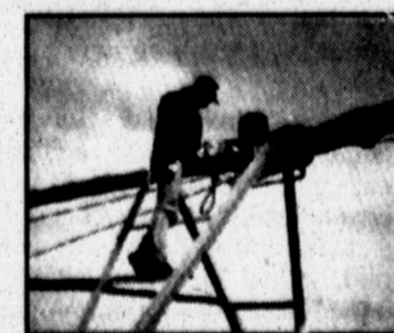
Checking the tower control box for loose wires.
