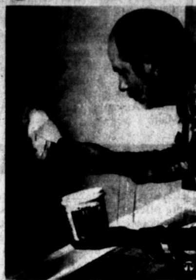
Repairing holes and cracks in walls and ceilings can be a quick and easy job.
