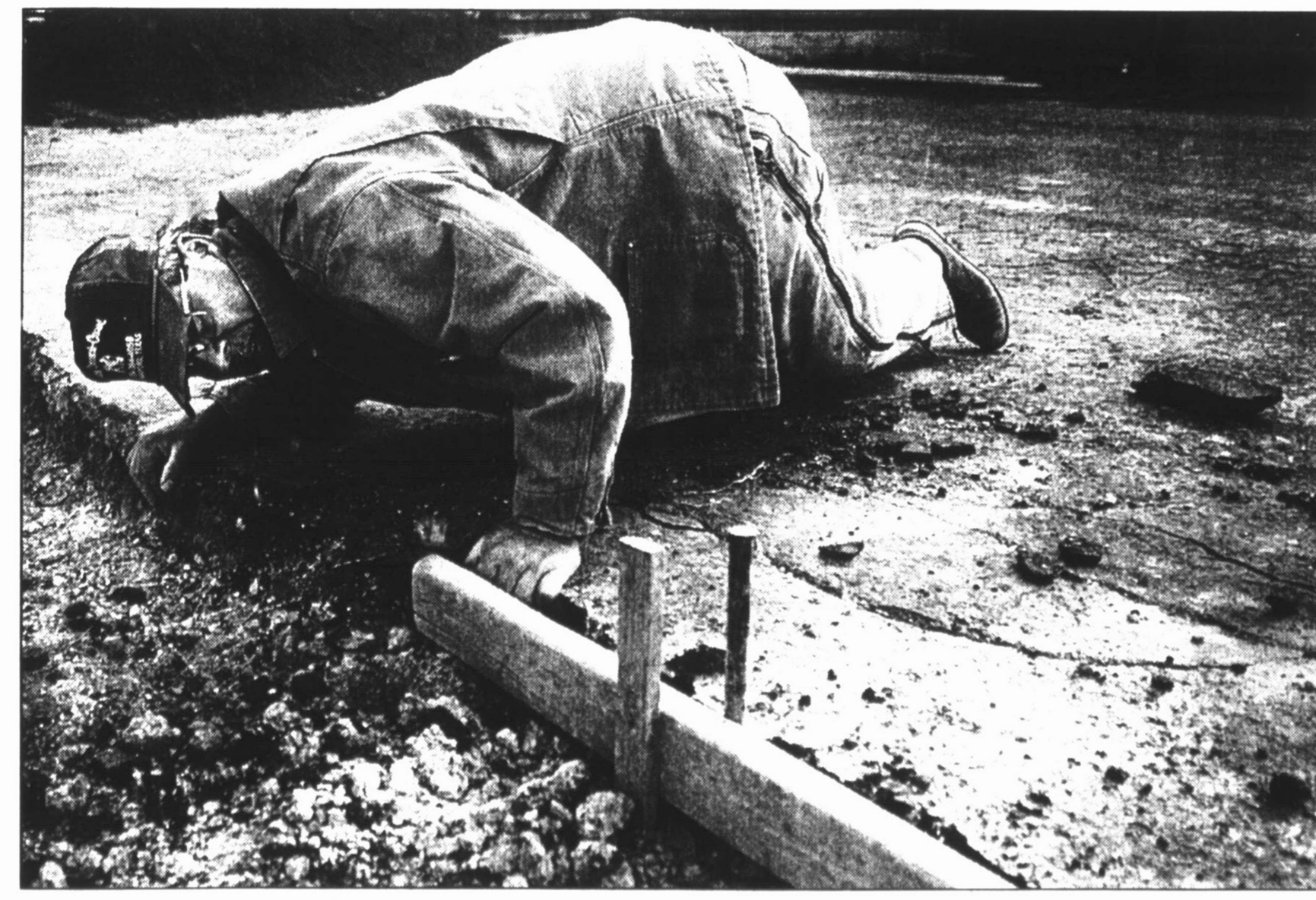
Work starts on funeral home facility Remodeling work has started on the Lone Star Insurance building at 601 Main St., where a new funeral home will soon open in Hereford. Ruben Ramirez, local cement contractor, checks
