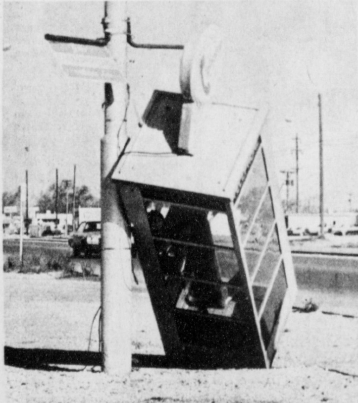
WIND DAMAGE.....High winds for the past several days have not only caused sinus sufferers more pain, but have caused some damage in the area. Muleshoe has reported gusty winds most of the past week with dust filling the air and cutting visibility down considerably. This telephone booth on West American Blvd. was apparently blown over by the high winds as were several signs in the city.
