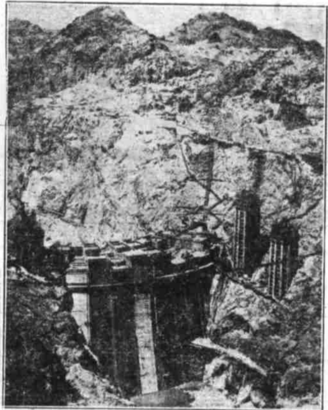
This view of Boulder dam on the Colorado river from upstream shows the mighty structure nearing its full height. The photo was taken by the bureau of reclamation when construction had progressed to 450 feet above the base. In the picture may be seen the huge intake towers through which water for the power and control systems will flow. (Associated Press Photo)
