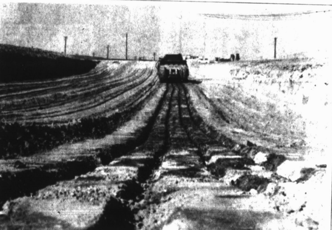
BIG SWEEP — This J619 "scraper" being used at the construction site of the new Wilson & Co. packing plant is one of two being used for the excavation of the basement of the plant's main building. The scraper is capable of picking up 21 yards of dirt in a single sweep. See story inside.
