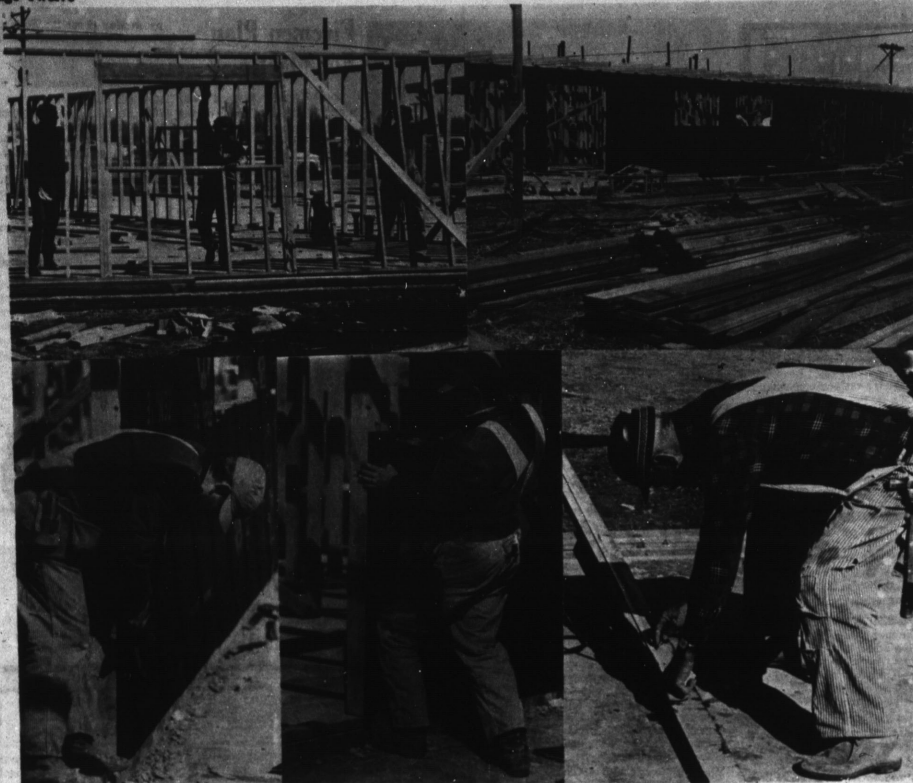
GOING UP FAST — The new El Dorado Arms complex, being constructed across from Sugarland Mall is taking shape rapidly. Already, the walls are in place, and workmen had started work on the upper level of the building by late Saturday afternoon. June 15th is the completion date for the construction.
