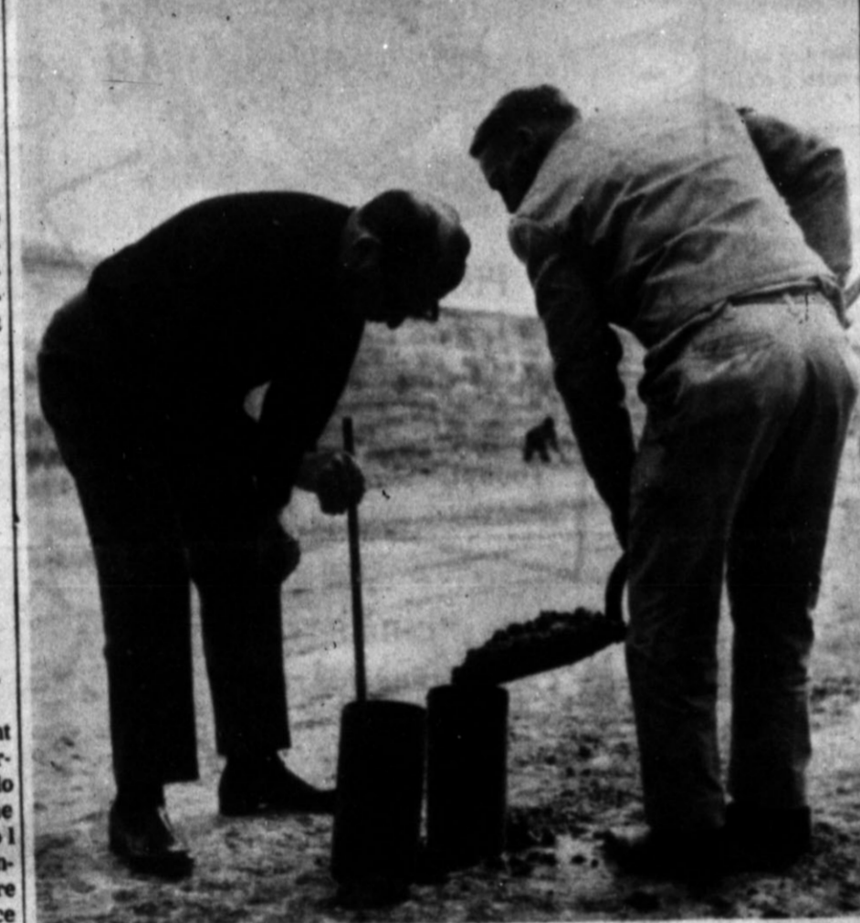
WORK CONTINUES on the new multi-million dollar Wilson & Company meat packing plant located about 3 miles southwest of Hereford along U. S. 60. Shown at lower left is former Hereford Mayor Ray Godwin who now lives in Amarillo and is District
