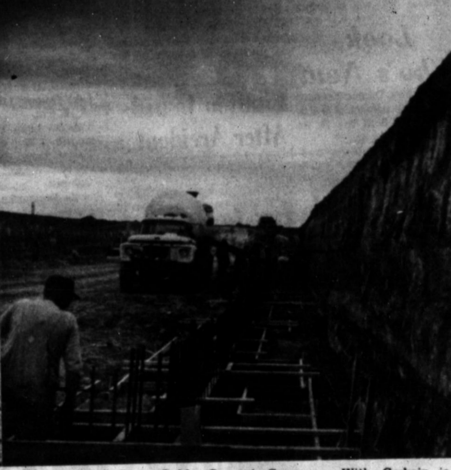
Manager for Crowe-Guide Cement Company. With Godwin is Ray Evans, an employee of the Hereford plant of Crowe-Guide. The men are making a cylinder test to see if concrete will meet required specifications. —Staff Photos
