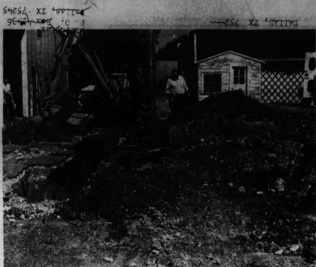
Accident Site Rescue crewman Gerry Hollinger inspects the ditch where Danny Gallardo suffocated while trying to dislodge a rock from a sewer line just east of Hereford Ford Lincoln Mercury. Gallardo, 25, fell into mud and water when the west side of the five-foot deep ditch caved in on him.
