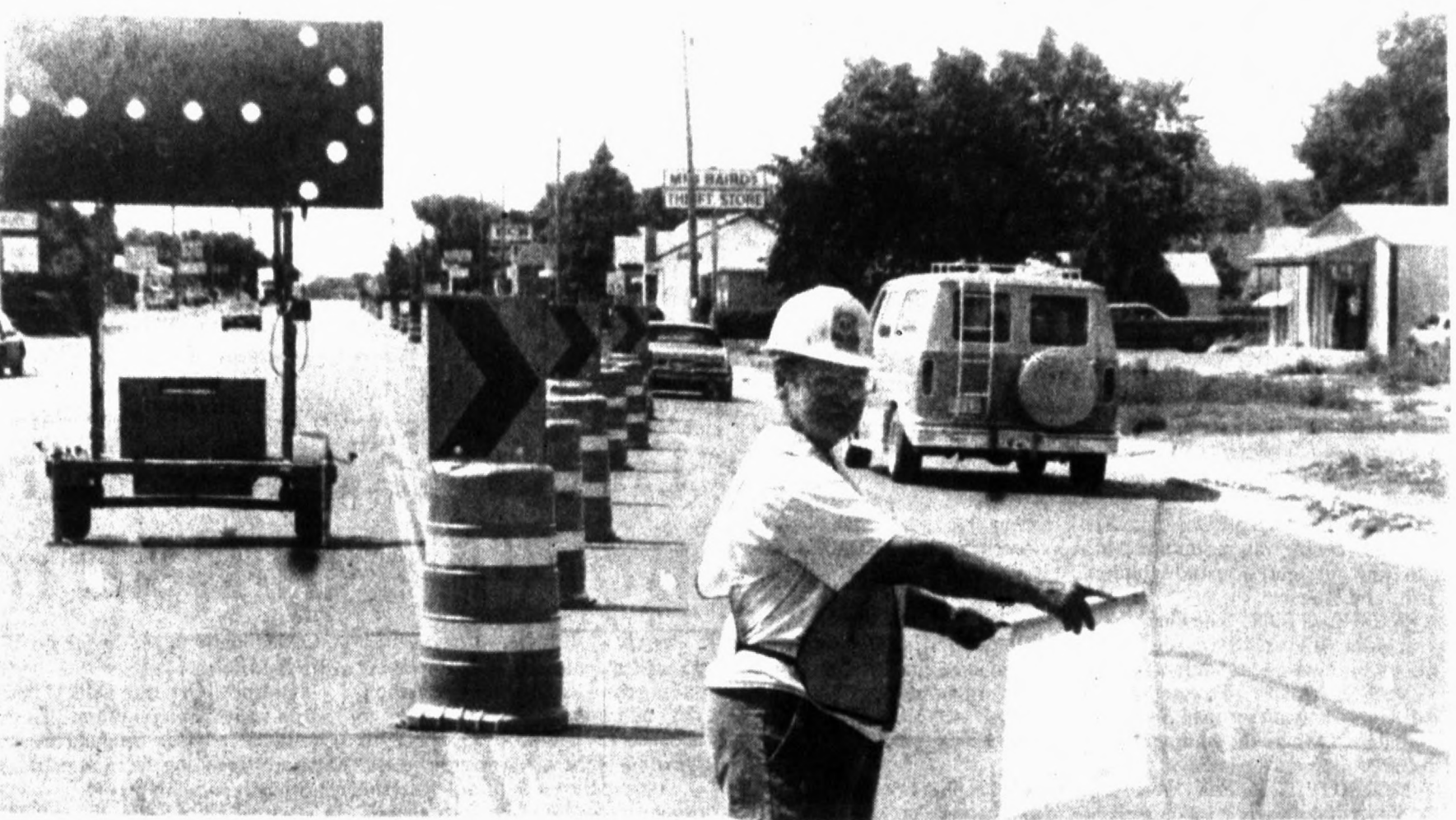
You've gotta go thataway Jeannie Whitacre of Amarillo directs traffic around one of the many orange traffic barriers on U.S. Highway 385 in Hereford recently. Gilvin-Terrell Company of Amarillo is reconstructing the highway, and the project will continue through October.
