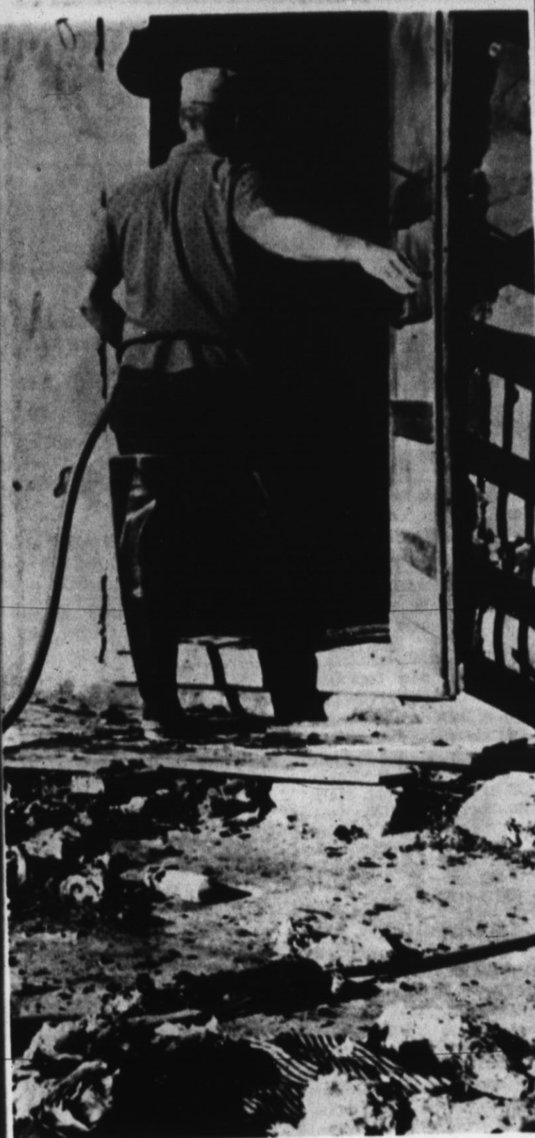
LABOR CAMP BLAZE — Firemen answered a call at the Labor Camp about 7:40 Wednesday morning. The blaze gutted a bedroom in the 4-room house, and apparently was caused by smoking in bed, firemen said. Firemen also had calls to a wheat fire and two small house fires this week. (Staff Photo)
