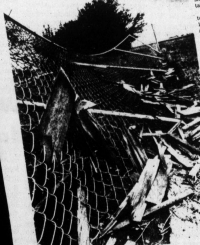
Possible Tornado Damage
