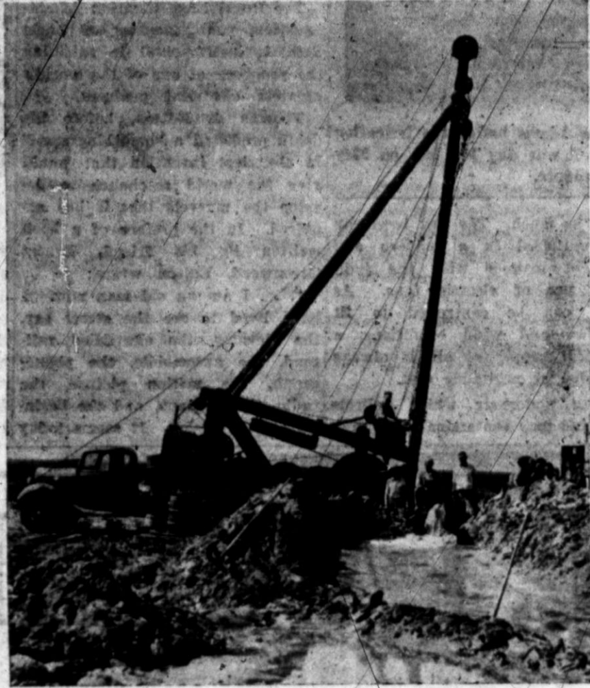
Plenty of sand, and plenty of water. They go hand in hand, according to W. W. Hill, who this month completed his new well shown above. This is the second well on his place, north of town on 25-Mile Avenue. The new 300-foot well is pumping a full stream.
