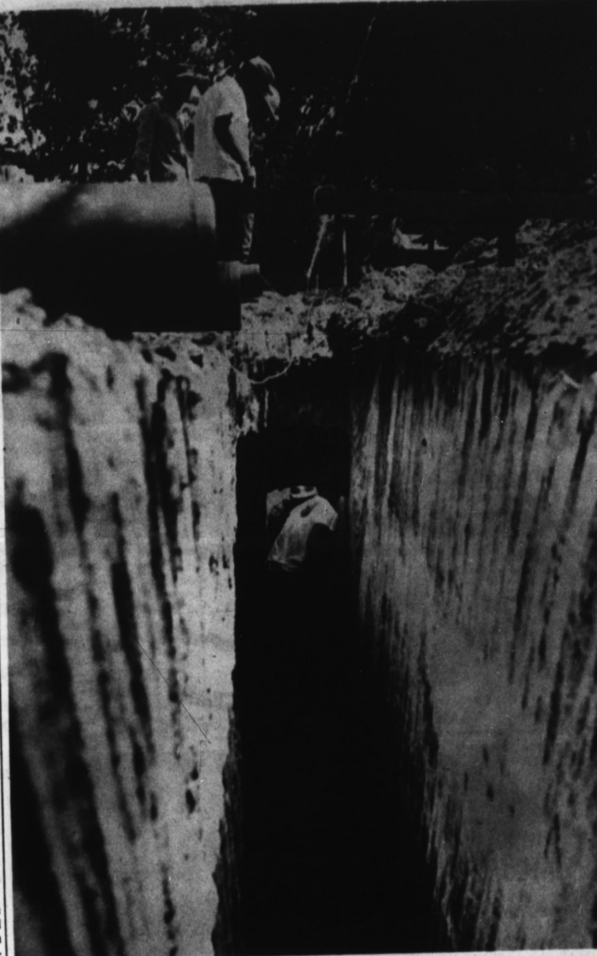
DOWN TO EARTH WORK — Workmen got down to business—about nine feet down— Tuesday as work continued on a main water and sewer line in north Hereford. The project is underway on 13th St., at the rear of the Sugarland Mall Shopping Center. (Staff Photo by Wain Miller)
