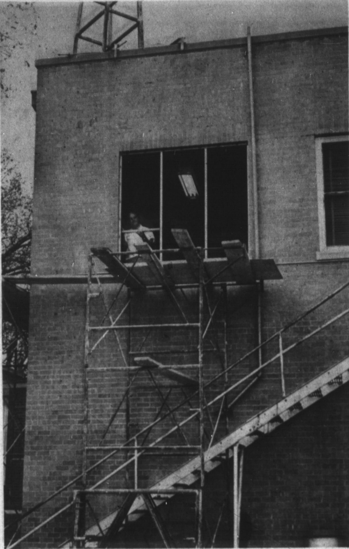
NEW WINDOWS — Construction began this week on installing the new aluminum windows on the second floor of the city hall. This picture was taken from the police chief's office. Hereford Glass Company was awarded the contract for the installation of windows. The windows will cut heating and air conditioning costs in the city hall, it is expected.
