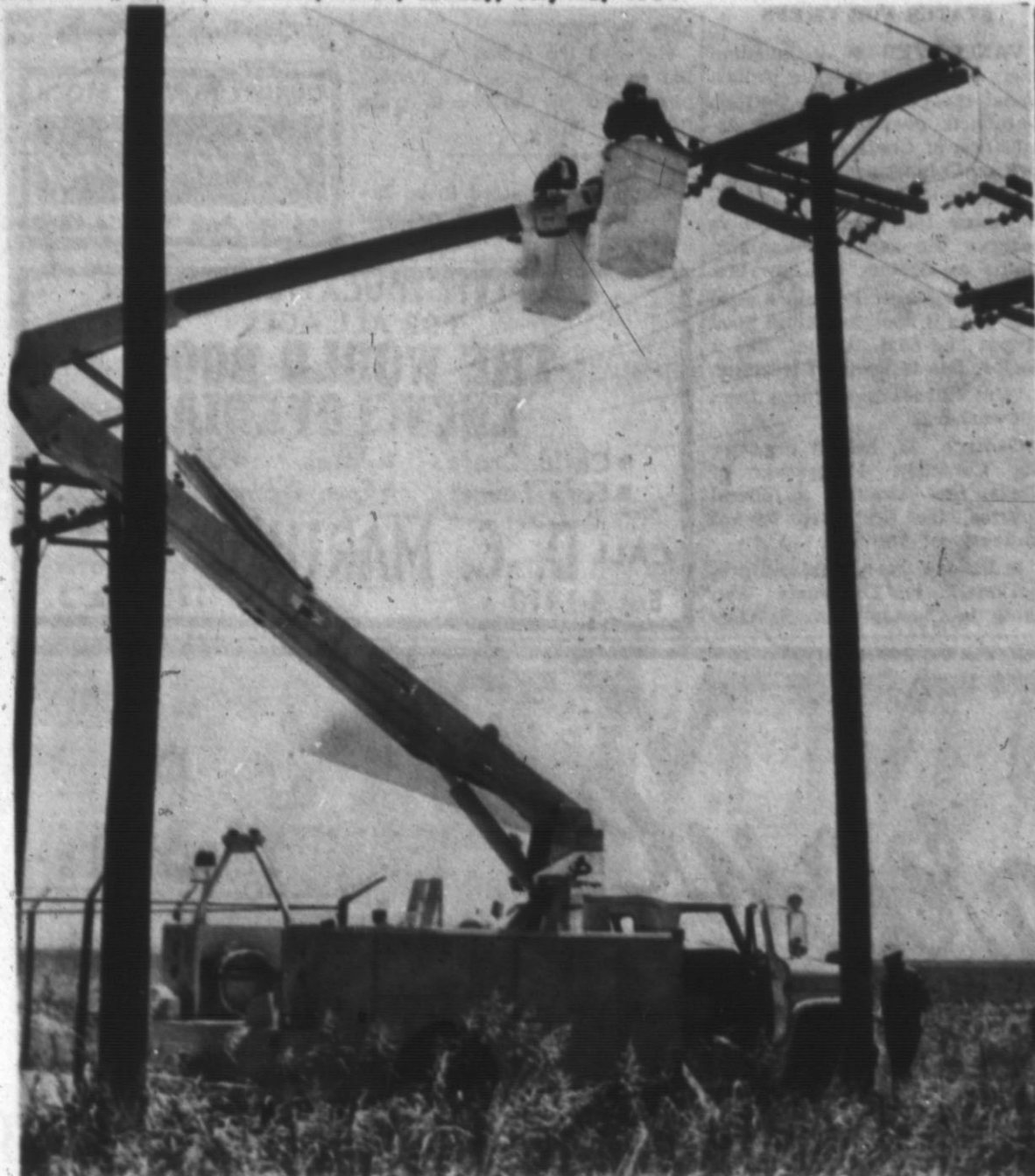
ON THE JOB — Linemen for the Deaf Smith County Electric Cooperative are shown here with the new $30,000 hoist truck in use, replacing the bolt-type clamps on the rural lines in Deaf Smith, Farmer and Castro counties. These men are working with a "hot" line as service was not interrupted during the switching of the clamps. (Brand Staff Photo)
