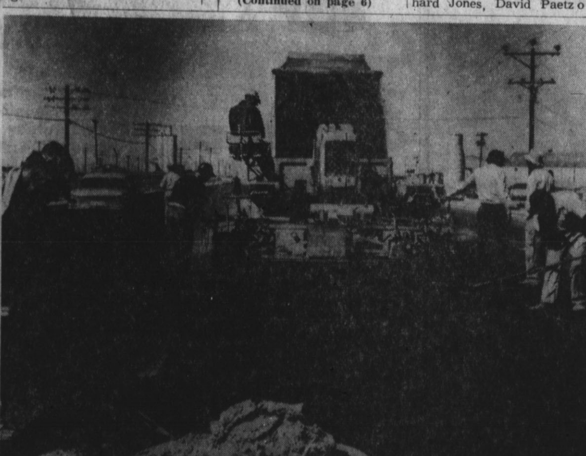
NEW PAVING started going down on east First Street this week, as the big expansion of U. S. Highway 60 inside the city limits nears completion. Engineers said the hot mix paving would be completed from the east city limits to Main Street this week and that the entire city portion should be done by mid-May. (Staff Photo)
