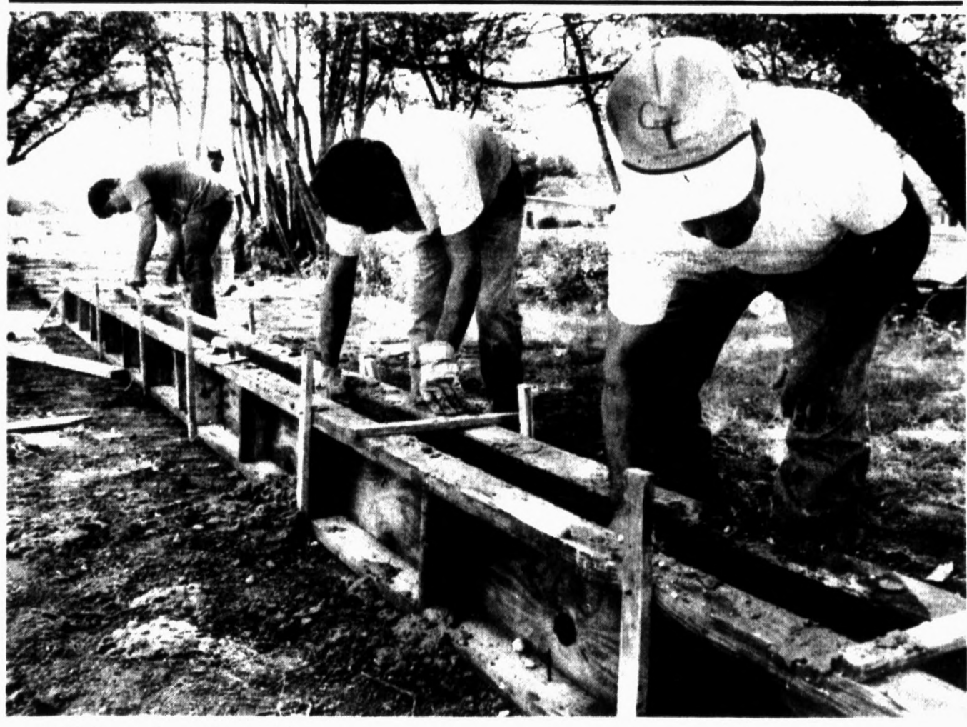
All in the family Elipolito (foreground), Rick (center) and James Garcia all do their fair share Thursday as Garcia Bros. Cement Contractors float concrete curbing as part of the city's improvement project at Dameron Park.
