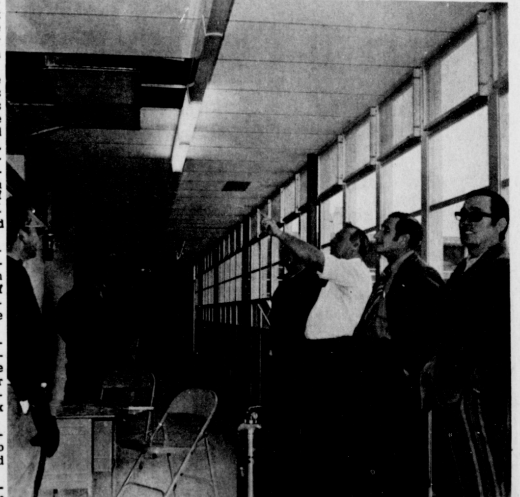
SMOKING HEATER . . . School officials and members of the Bailey County Volunteer Fire Department are shown looking at the vent from which a great deal of smoke came through at the Mary DeShazo Elementary School Thursday morning. A transformer on a heater central system burned and the smoke was drawn into the building. Several units of the Fire Department were called out for the early morning alarm.
