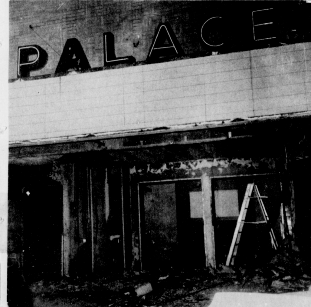
REMODELING BEGINS . . . The old Palace Theatre on Main Street is being completely remodeled and will be the new location for Gordon Wilson Appliance. Wilson reported that the building will contain approximately 3,000 feet of floor space which is considerably larger than his present location. Wilson estimates that it will be at least the first of April before he will be moved into his new location.
