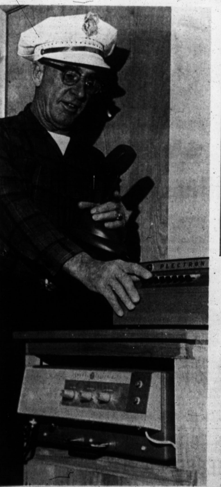
DEMONSTRATING THE OPERATION of the base station for the radio fire alarm system now in operation is Clay Angelo, fire marshal.
