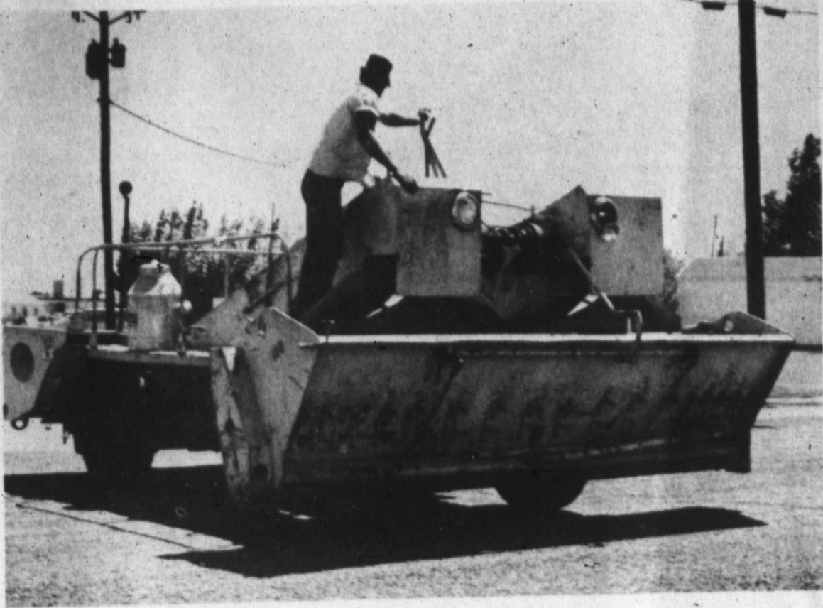
BUSY ON PARK AVENUE last week was this gravel spreader, being used by an Odessa contractor to put a seal coat on Park Avenue and Harrison Highway. The coating of asphalt and gravel will help prepare the roads for the winter moisture. (Staff Photo)
