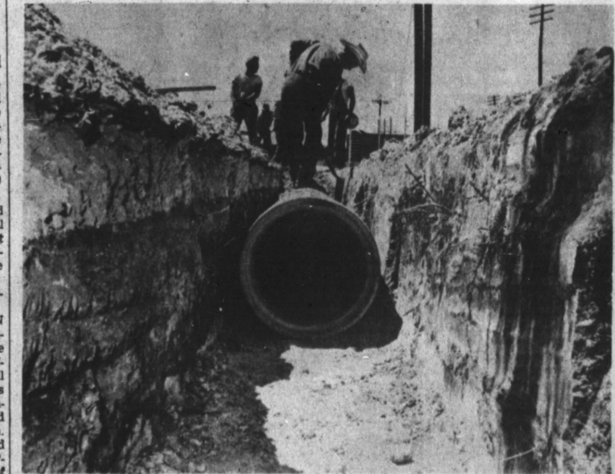
PREPARING FOR THE STORM, the city of Hereford is installing large storm sewers along Park Ave. This sewer is being installed from Park Ave. along Ave. K to Highway 60. Plans include installing another from Ave. E and Park Ave. southwest to Dameron Park.
