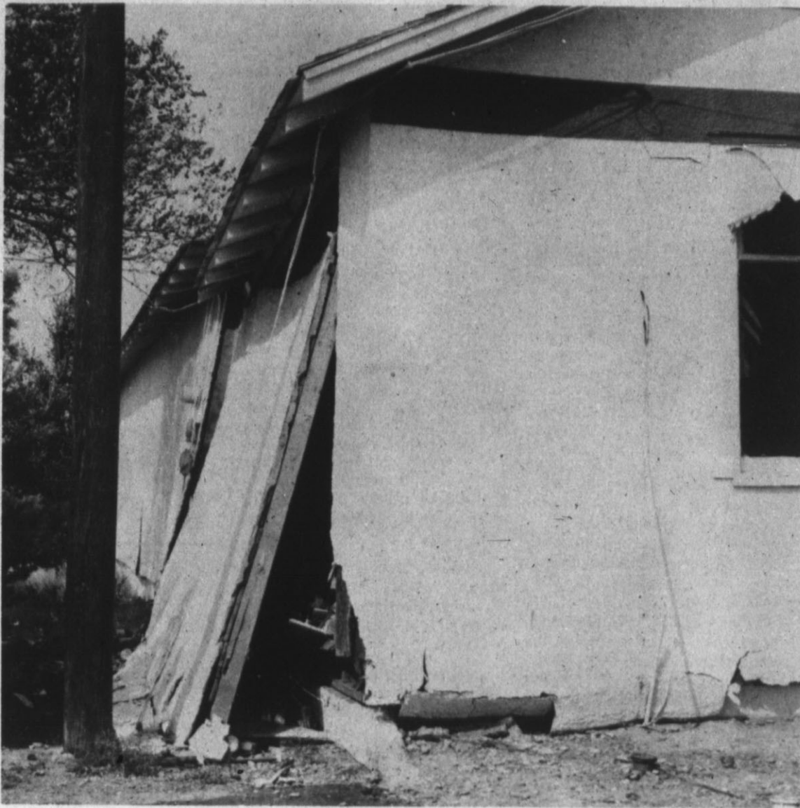
DAMAGED PORTIONS of the Westway Store are shown following an explosion which rocked the structure Friday afternoon. Canned goods and other merchandise spilled onto the ground as debris was thrown over a wide area. Considered a total loss,
