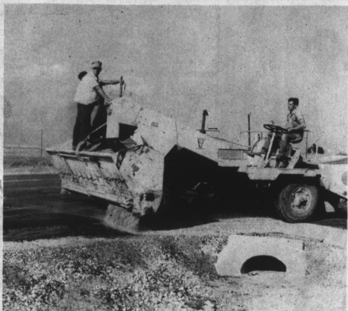
FINAL TOUCHES of the new four-lane road to be finished up this week. Traffic will be kept on one side for another week before it is turned loose on the new road. (Staff Photo)
