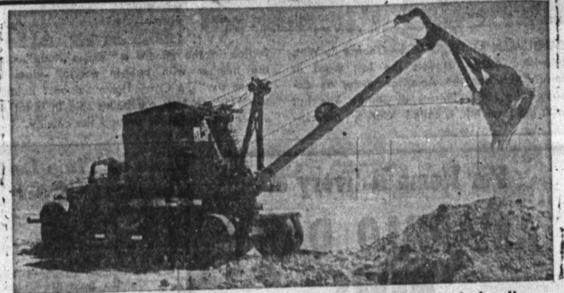
We've added new equipment now, a back-hoe and dragline, to handle your slush pit clean-out and other specialized digging.
