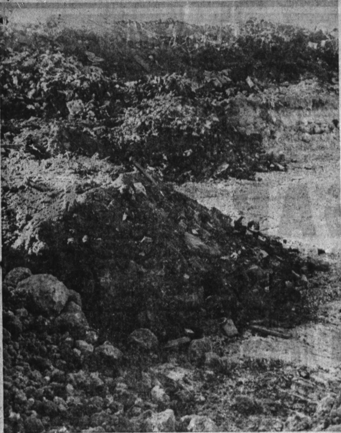
NEW SYSTEM —Part of the city's plan to improve the looks of the old dump grounds east of town is shown above. The object is to dig a trench, scrape the trash presently standing on top of the ground into the trench, and cover it over. Portions of the area have already undergone the treatment, and the rest will soon be completed. After the entire project is finished, one trench will be maintained for county dumping at all times. The city's refuse will be taken to the new dump site, being operated on the same plan of digging, dumping and covering, presently. (Staff Photo)
