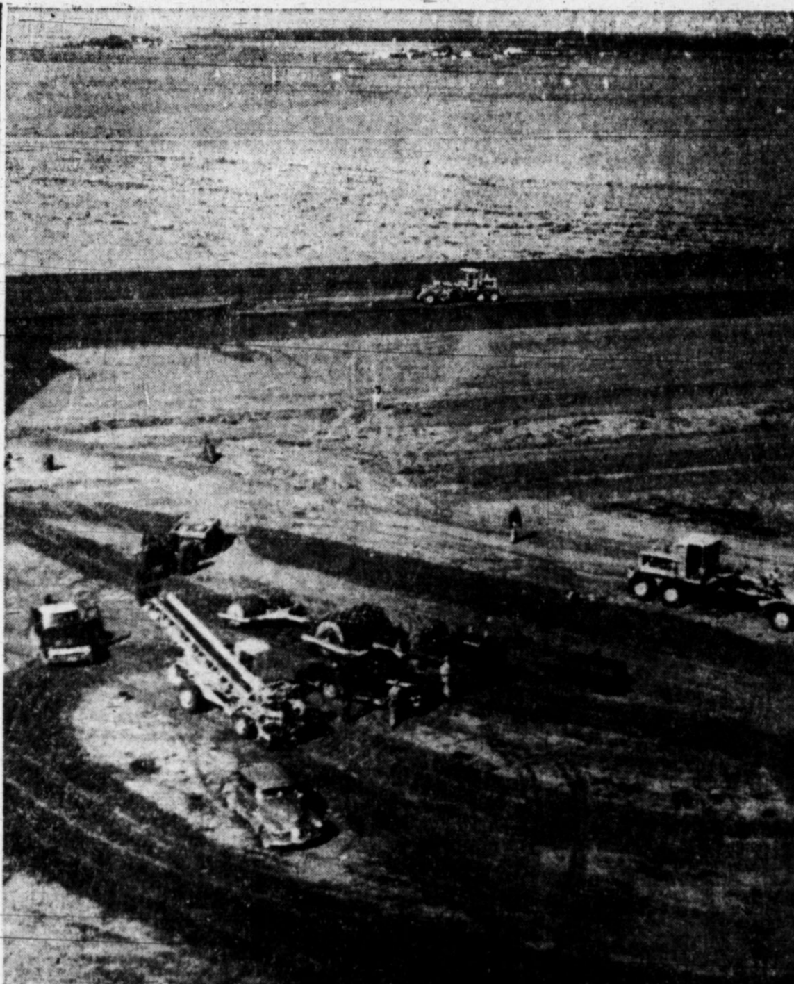
DIRT WORK CONTINUES —While rain has hampered work on the runway and taxi strip of the new city airport, the moisture has also helped in compacting the subsurface. Crews and machines, above, have taken advantage of breaks in the weather to keep some work going. An all-weather landing strip will be completed soon, but asphalt topping of the airport facilities will be postponed until next spring. (Staff Photo)
