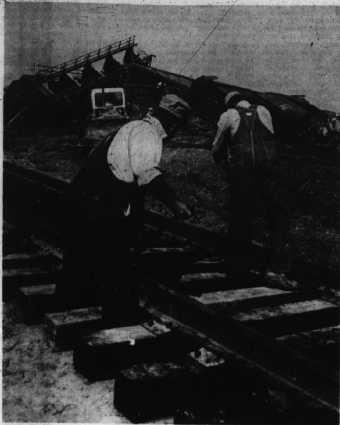
WORK CREWS INSTALLED a temporary by-pass line around the wreckage of an east-bound Santa Fe freight. Forty cars of the train stacked up and splintered like match-boxes due to a faulty journal about 12:30 a.m. Friday. Damages are expected to be
