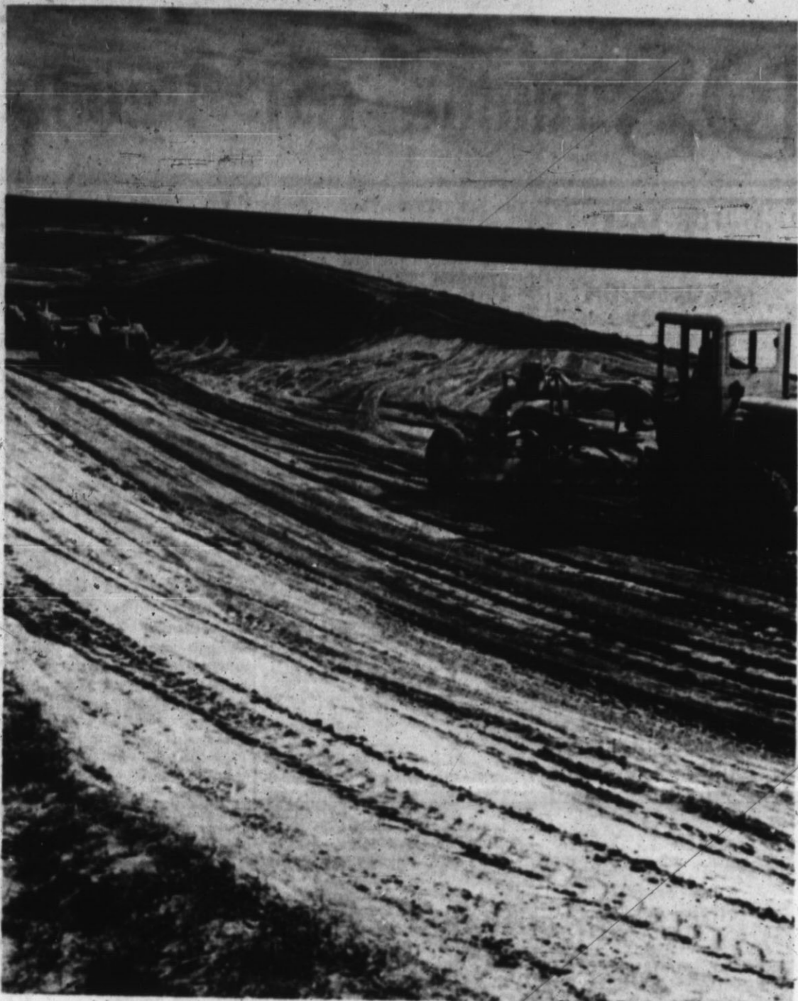
FOLLOWING THE HEAVY rains of the past two weeks which sent flood waters swirling down Frio Draw, work was again underway to strengthen the dam on the Harlan Frye farm, south of Summerfield. As heavy rains saturated the area, water flowed around the ends of the dam and, over the top. However, the earthen structure held. (Staff Photo)
