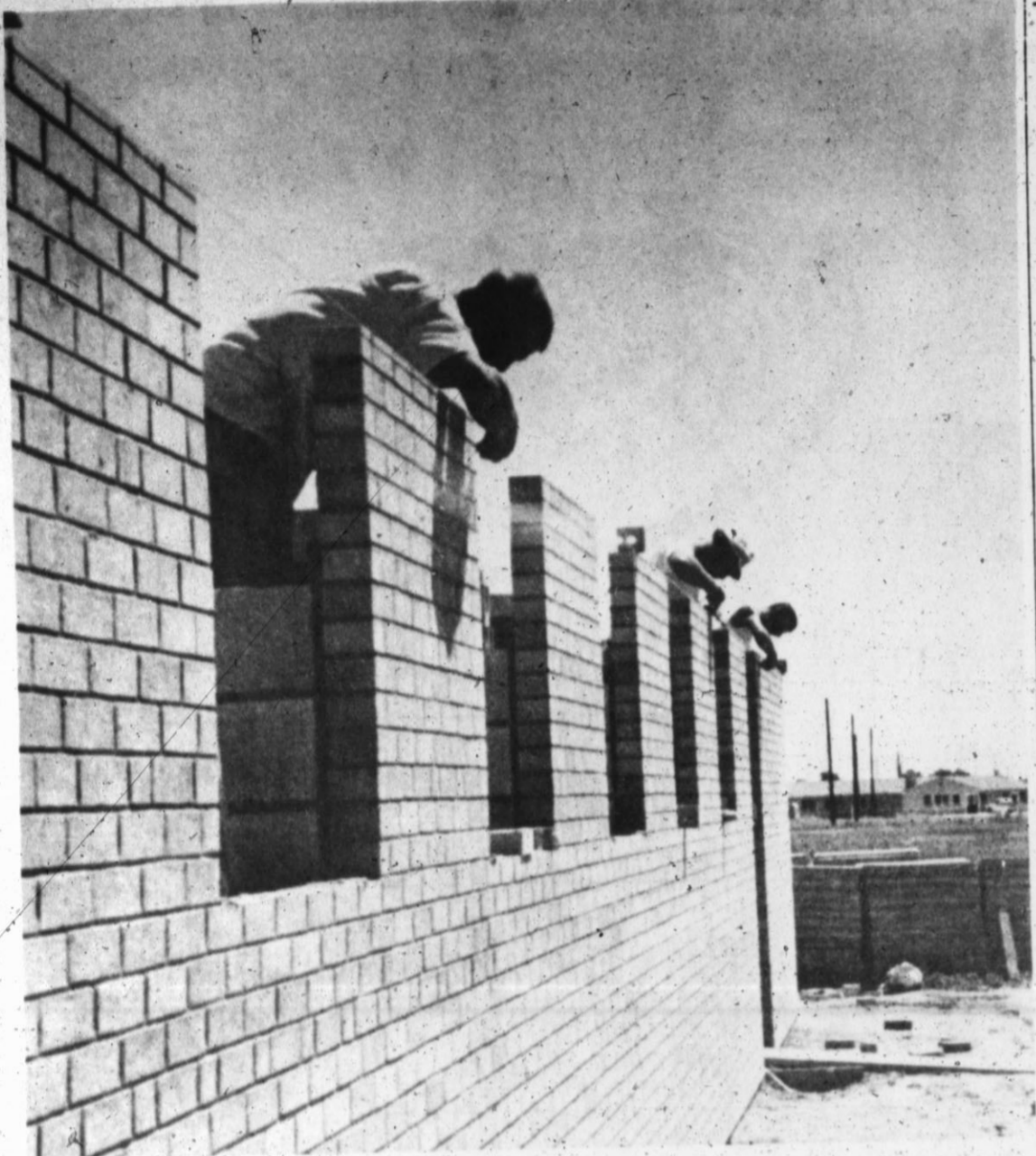
BEGINNING TO TAKE SHAPE, the new field house for the high school football field will be completed in time for the first home football game in the fall, if the present work rate keeps up. The field house will include dressing rooms and public restrooms. (Staff Photo)
