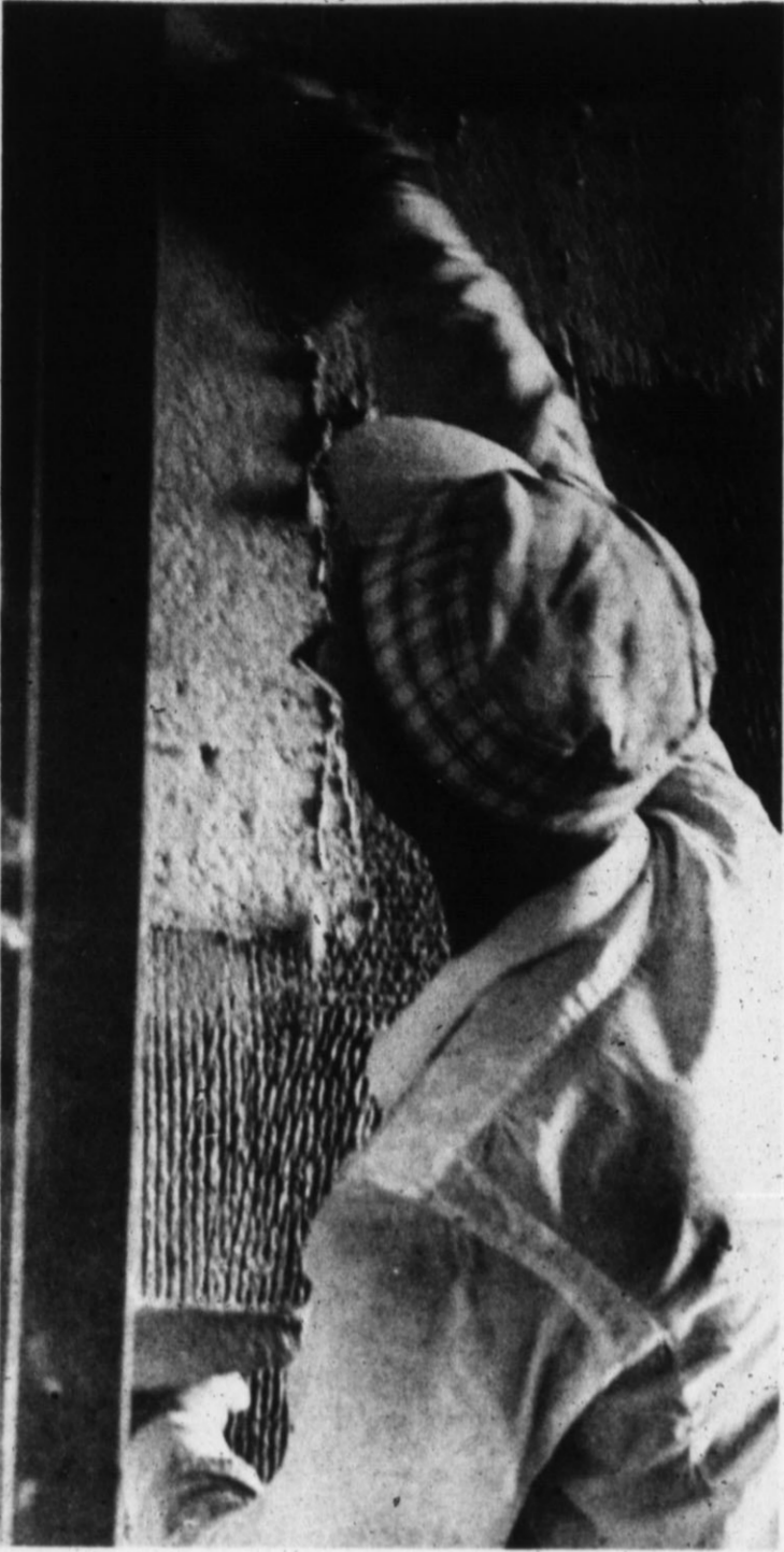
PLASTERERS APPLIED finishing touches to the structural work on the first unit of Kings Manor here this week. The first unit of the Methodist retirement home is slated for completion in September, with work on another unit scheduled to be underway by that time. Bids for a nursing unit will be accepted in the near future. (Staff Photo)
