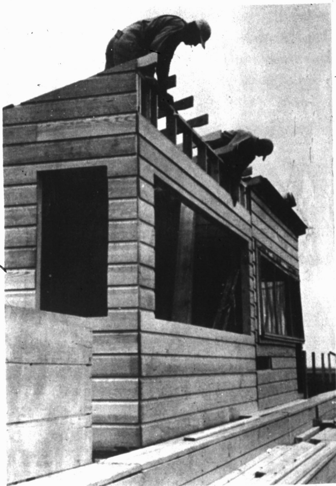
AN ADDITION TO THE PRESS box at the new high school football field began to take shape here last week as work continued in preparation for the first home game Sept. 18. The new fieldhouse and gridiron are expected to be completed in time for the game, according to P. L. Stevens, superintendent of schools. (Staff Photo)
