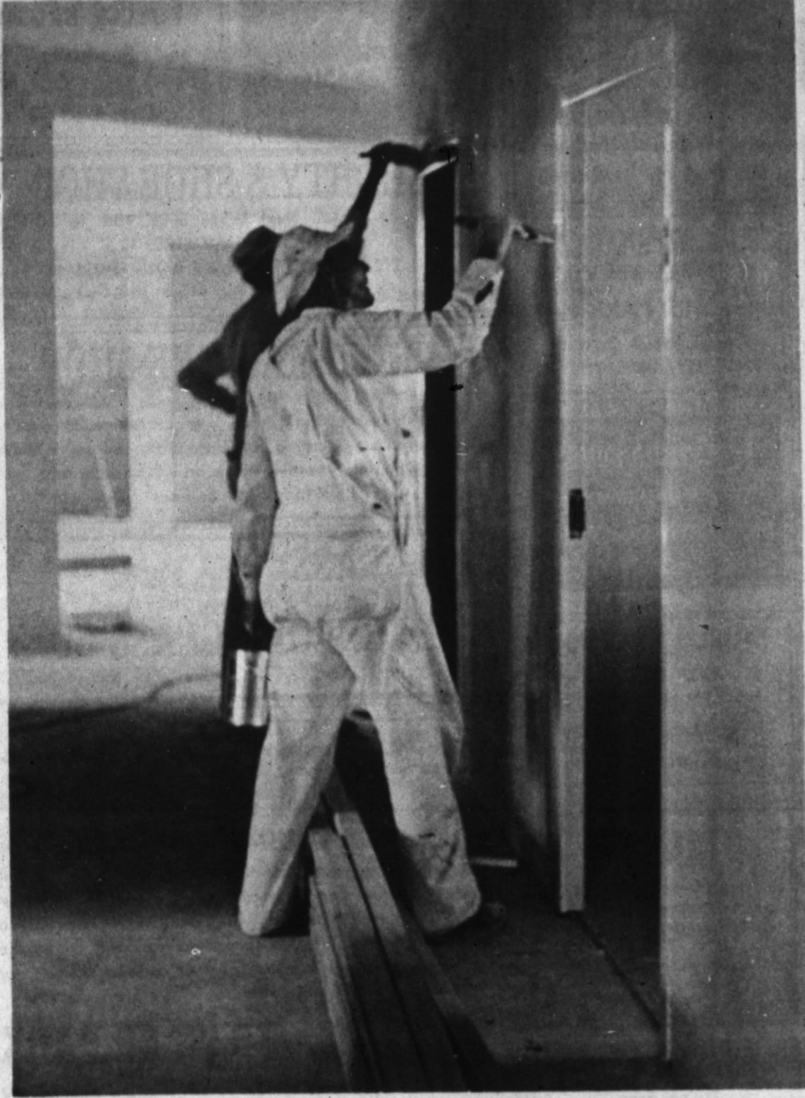
NEARING COMPLETION, Kings Manor received a coat of paint on the inside here last week. The Methodist retirement home is slated for opening in the fall, and work on a nursing care unit is slated to get underway then. Workmen were also installing tile and fixtures. (Staff Photo)
