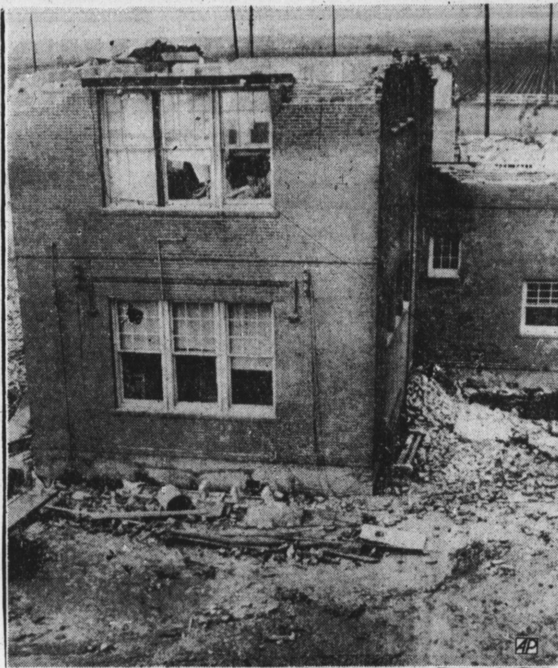
TORNADO HITS SCHOOL —The 41-year-old home economics building at the LaCoste Community near San Antonio was ripped by a tornado that hit the area. The tornado took off the roof and weakened the building. Supt. A. D. Blue said it probably would be condemned. There were no deaths. (AP Photo)
