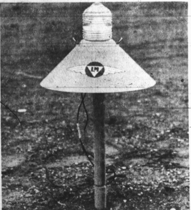
RUNWAY LIGHTING installation at Hereford Airport began Tuesday. Shown above is one of the 52 lights which will be installed along the full length of the runway. The "flying farmers system" of lighting is being installed by city employees. Conduits for the system are already under the runway. The lights will be in operation from sundown to sunrise. (Staff Photo)
