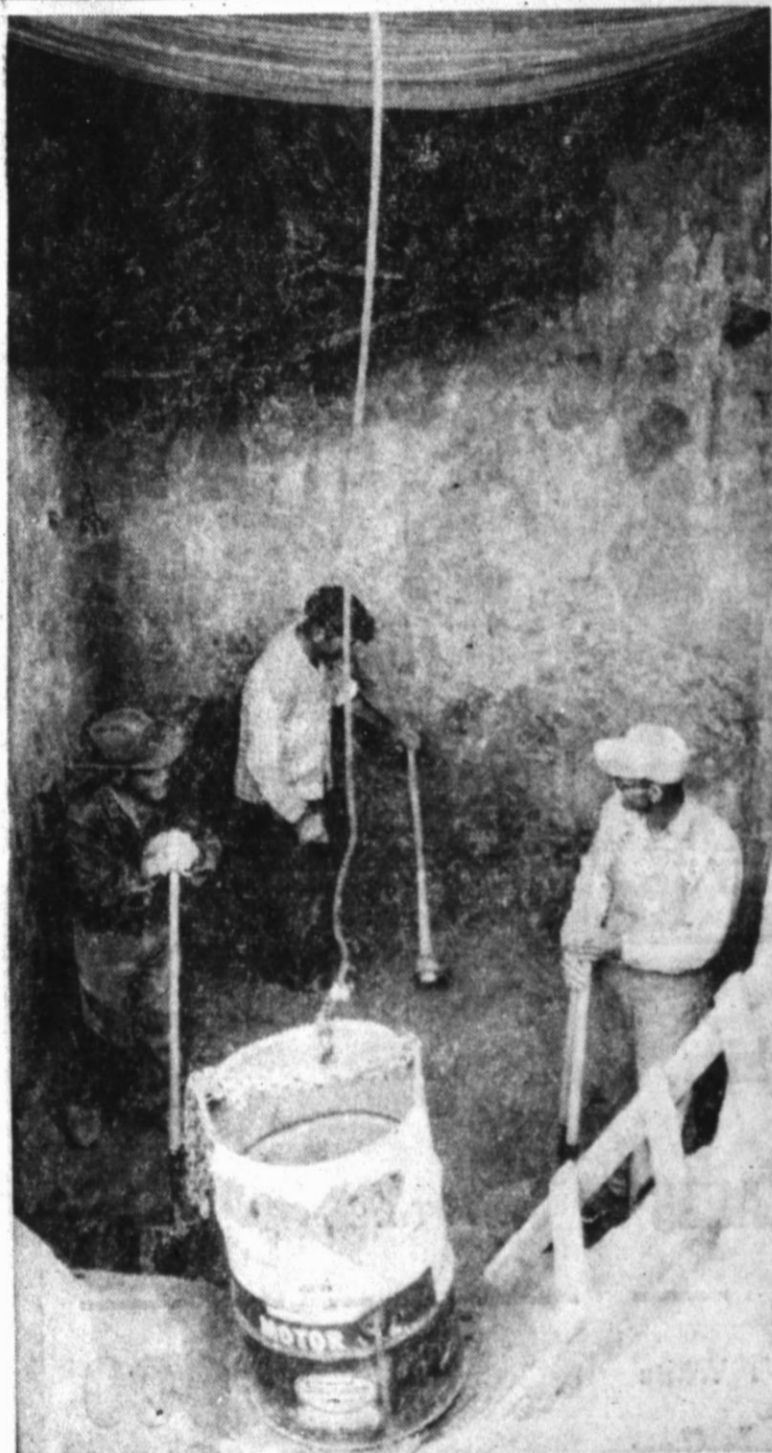
A PAUSE IN ROUTE—Workers on the new 600,000 bushel capacity grain storage unit presently under construction in the Sims community pause for a breather while digging a 23-foot hole where truck-dumping will take place. Though the workers were spared 10-feet of digging by a machine, they are shown here at 13 feet depth Wednesday afternoon. The rest of the way had to be done by hand. (Staff Photo)
