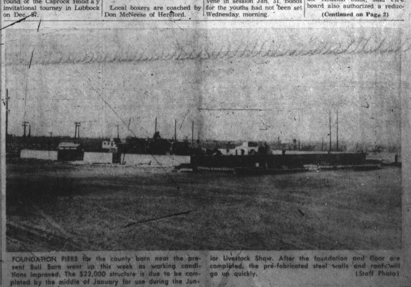
FOUNDATION PIERS for the county barn near the present Bull Barn went up this week as working conditions improved. The $22,000 structure is due to be completed by the middle of January for use during the Junior Livestock Show. After the foundation and floor are completed, the pre-fabricated steel walls and roof will go up quickly. (Staff Photo)
