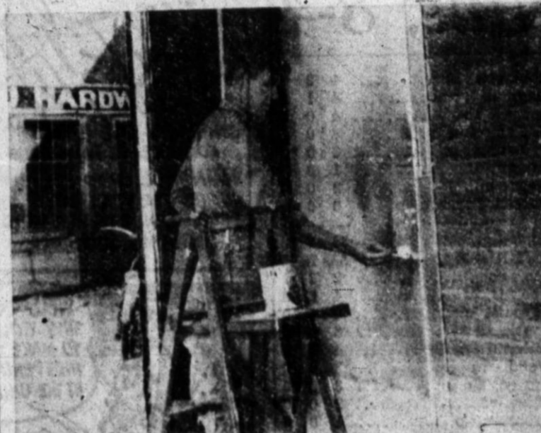
PICTURED HERE re-painting a steel door, Eugene Miles has been employed by the Star theater for almost four years —Brand Staff Photo.
