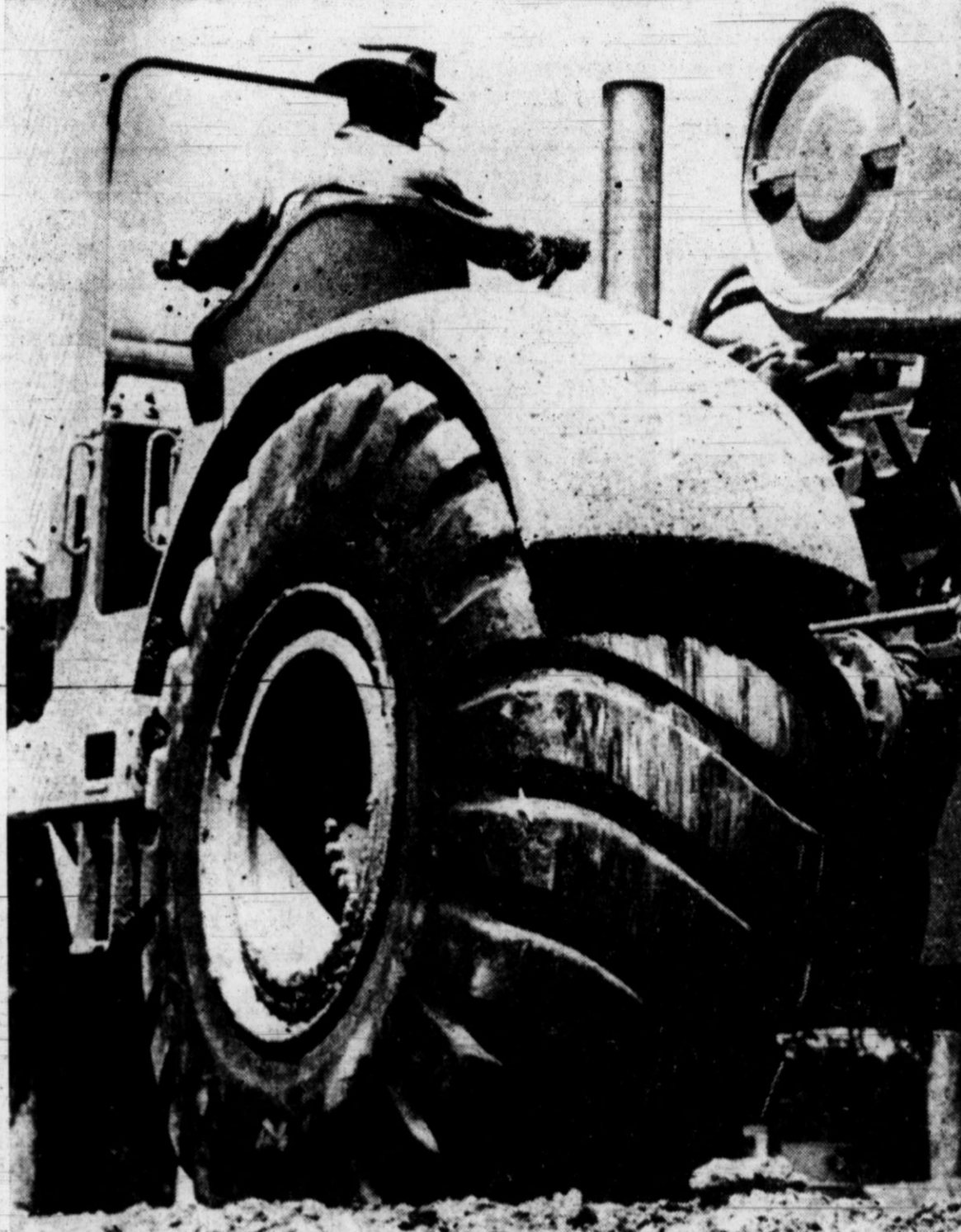
BIG WHEELS TURN—A driver of a mammoth steam tractor, above, eases his machine along as it takes a 20-ton bite out of the surface of Highway 51 in Hereford. Work by crews employed by contractor Ivan Dement were proceeding this week with grade leveling of the road, scheduled now for completion from Highway 60 north to the city limits in late September. (Staff Photo)
