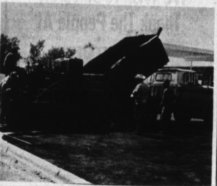
WORK CONTINUES — Workmen apply a layer of asphalt to the driveway of the new Mobile service station being built on North 25 Mile Ave.
