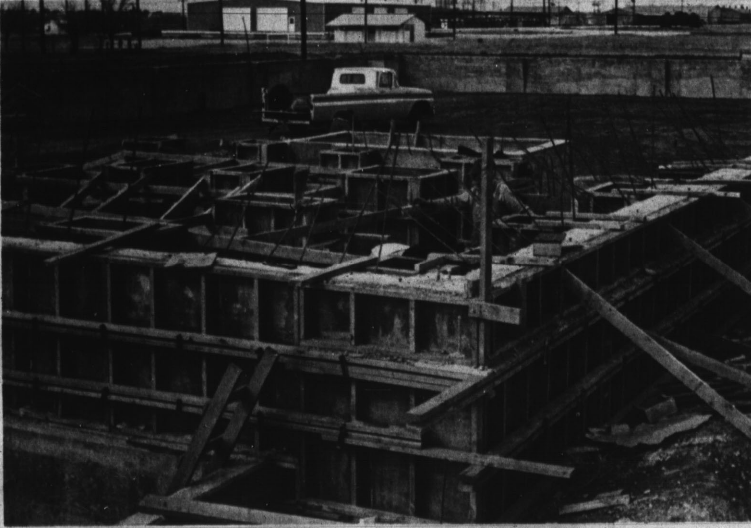
PROGRESS REPORT — Co-concrete forms and foundation work have begun on the $300,000 Swift Mineral Feed Plant being constructed east of Hereford. The plant will employ about 20 people when completed and will distribute its feed product through several states in the mid-west. (Hereford Brand Photo)
