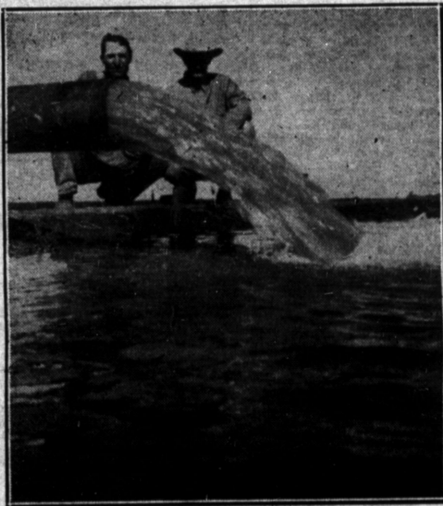
Above is pictured the irrigation well on the T. W. Roberson farm, 5 miles Southwest of Hereford. This well is in that part of Deaf Smith County where several attempts have been made to bring in good wells, but very few have been successful! This well was drilled by, and the FAIRBANKS-MORSE PUMP furnishing the water was sold by the BRADFORD SUPPLY CO. of Hereford. This well has been in operation constantly day and night for the past three weeks and is throwing more than 1200 gallons of water per minute.
