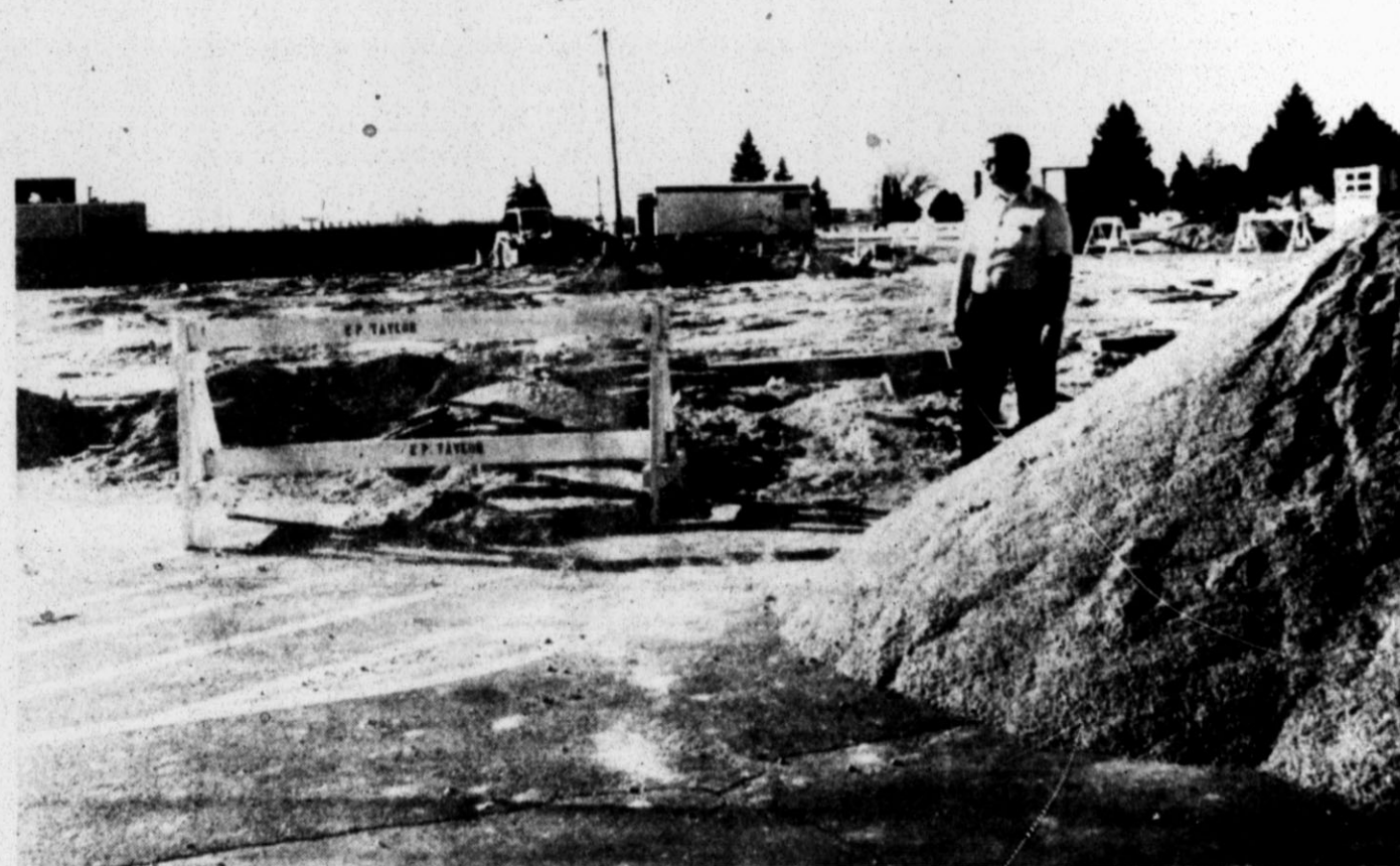
Store Addition Site TG&Y co-manager G.C. Hagle looks over the area destined to become a 20,000-foot addition to the west side of the department store. Work began recently on the addition and is due to be completed sometime in the spring, according to Hagle. The addition will bring the entire area of the store to more than 70,000 square feet and will make departments more accessible to shoppers. [Brand photo by Paul Sims]
