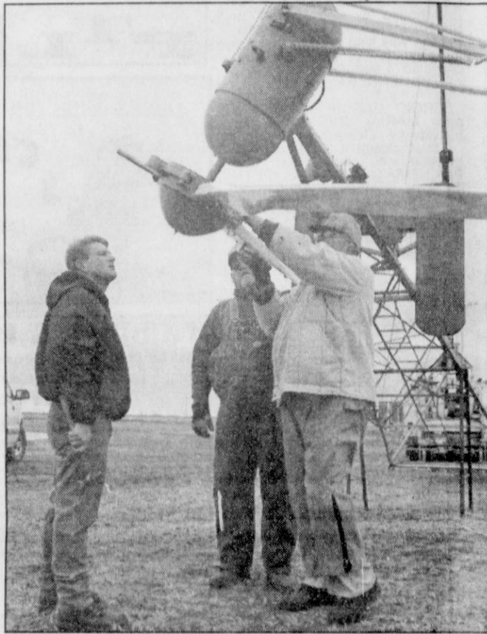
(Photo at Right) Rick Cazares of Panhandle Water Well and Jim Tope provided the equipment needed to raise the generator into position.
