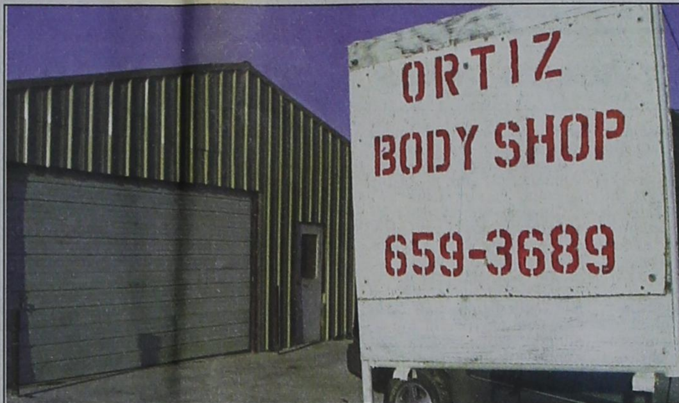
ABOVE: The window in the door of Ortiz Body Shop was blown out following a compressor explosion.
