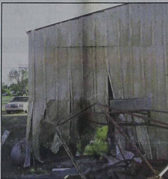
BELOW: An air compressor exploded behind Ortiz Body Shop on Monday night, September 29, 2008, damaging the building.
