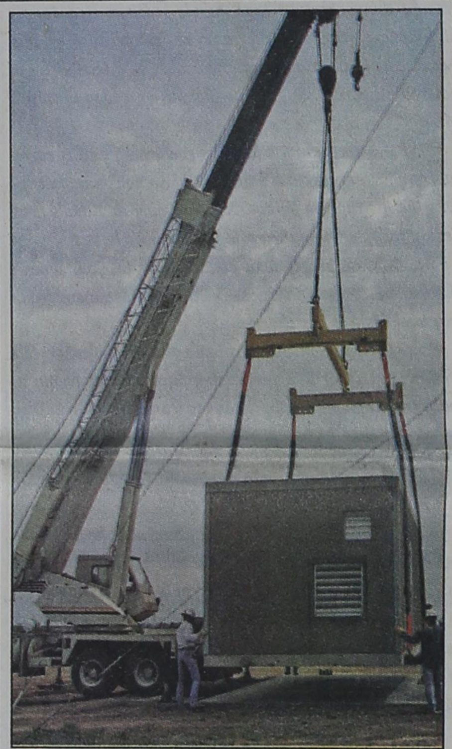
PTCI moves another step closer to providing telephone service over the cable television network in the city of Spearman as a crane lowers the new equipment building into place.
