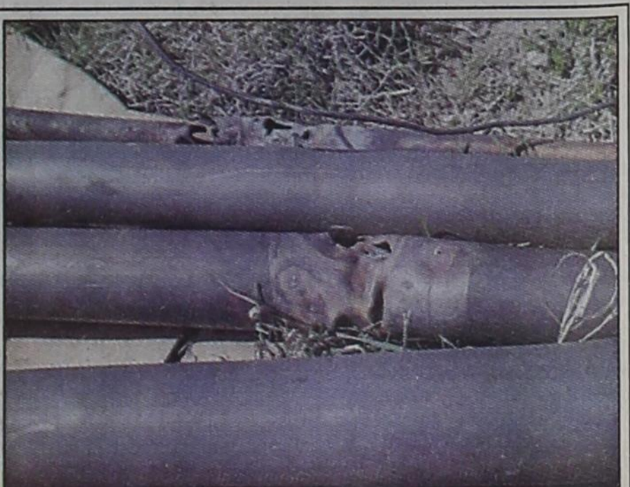
These copper inner bay lines were damaged when the KTOT tower was struck by lightning and the lightning burnt holes right through them.
