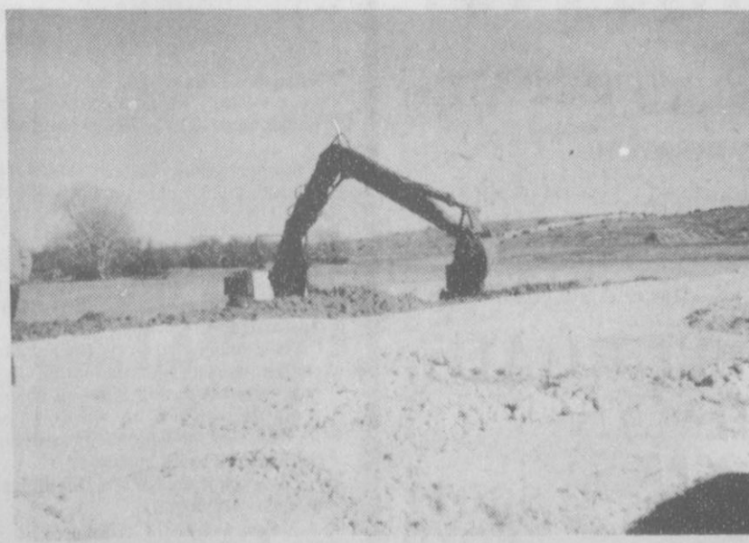
A heavy duty loader begins to scoop out dirt to start building the dam on Dec. 14, 1988.
