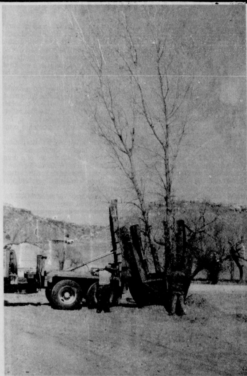
Workmen are replanting a tree in the park area behind the Palo Duro Dam. The tree was taken from a stand of trees in front of the dam.
