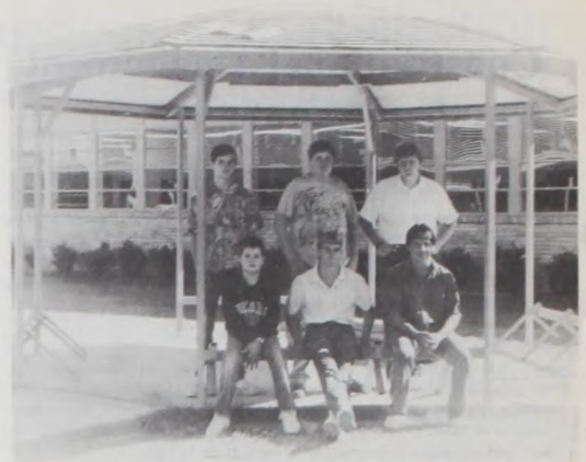
THE "GENERAL CONSTRUCTION PROCESSES" class of MHS is completing construction of a gazebo situated between the Junior High wing and the High School. This is a joint project of the school and the PTO. The gazebo consists of a metal framework with plywood decking covered by cedar shingles. Connecting sidewalks were also built by the construction classes. Rudy Koesler is the instructor. Class members include, l to r, sitting - Chad Bayer, Chris Klement, Weldon Hermes; back - Jim Herr, Danny Black and Mike Abney. Janie Hartman Photo
