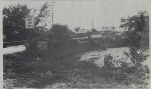
Evidence of damage from the flash flood.
