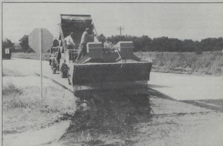
PUTTING THE finishing touches on newly paved S. Ash Street are Precinct 3 employees Billy Poyner and Wayne Trubenbach. The S. Ash/W. Eddy Street project was a joint effort of the City of Muenster, Precinct 3 and Precinct 4. Janie Hartman Photo
